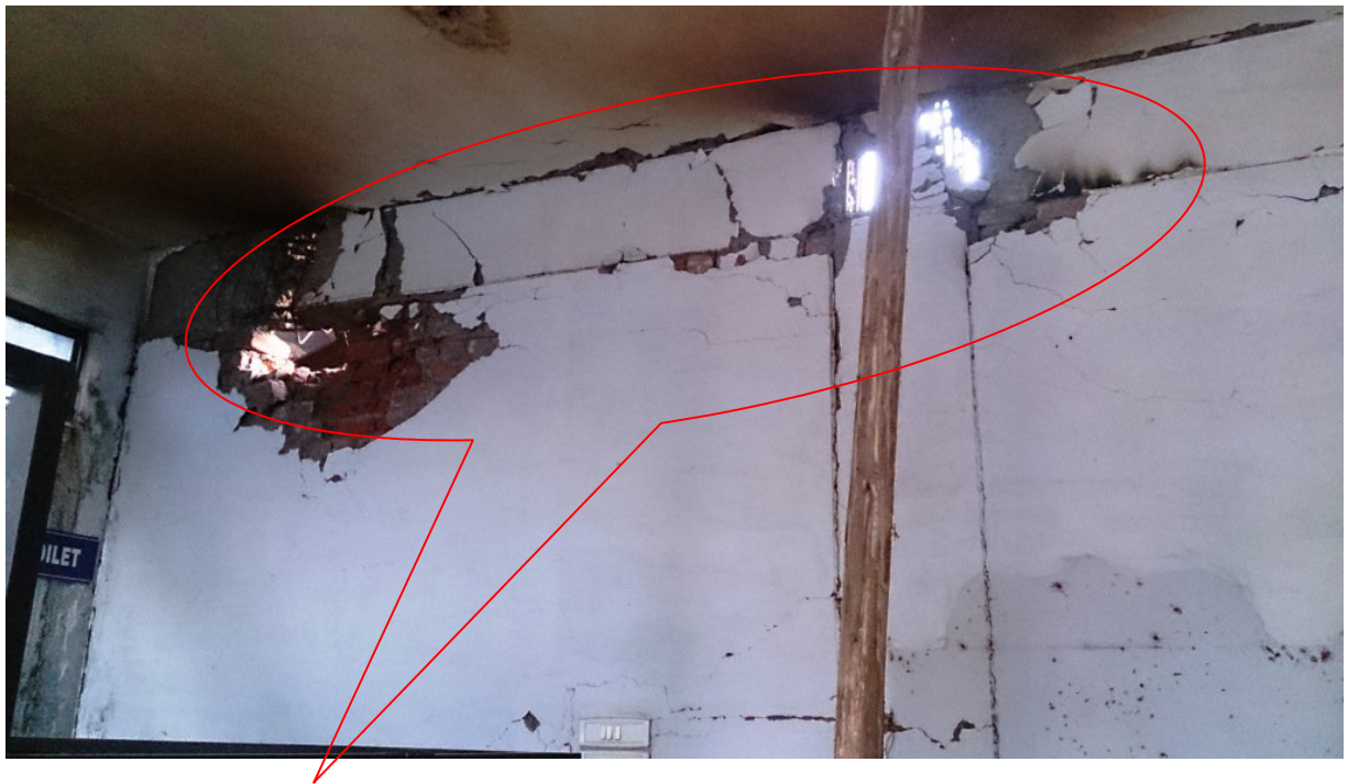
Cracks and spalling of concrete in the front portion of the building
