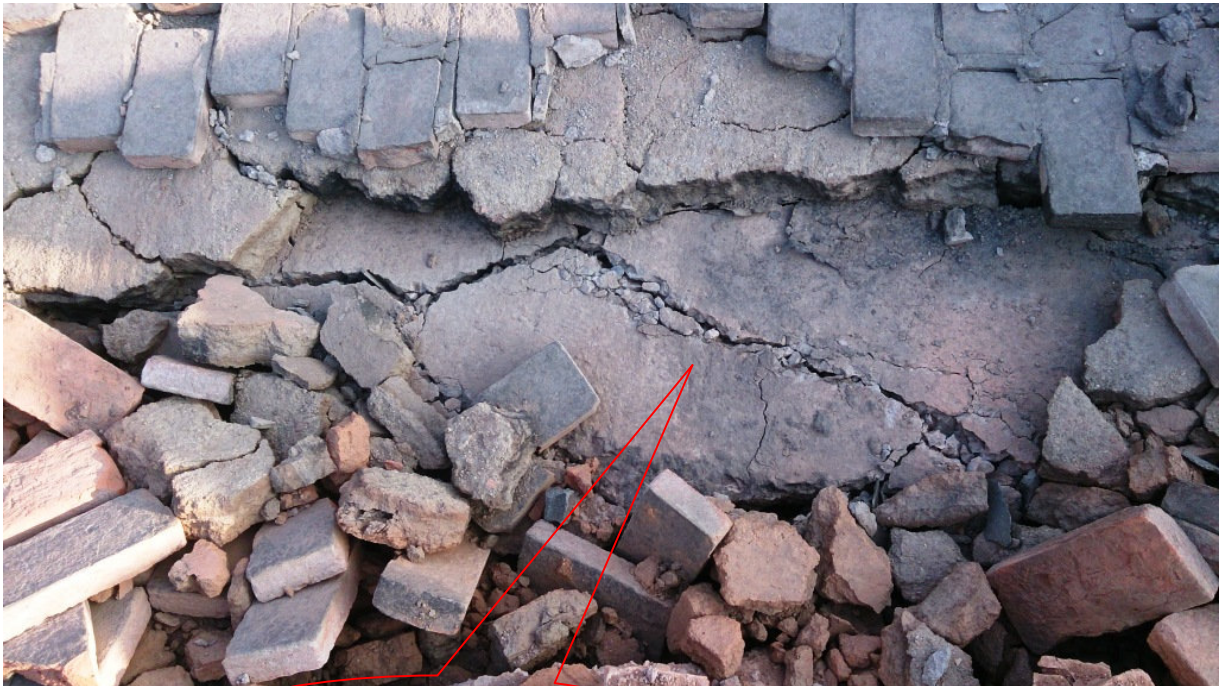
Softened concrete in the slab
