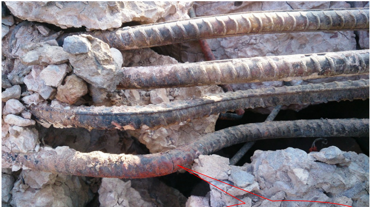
Crack in Rebar
