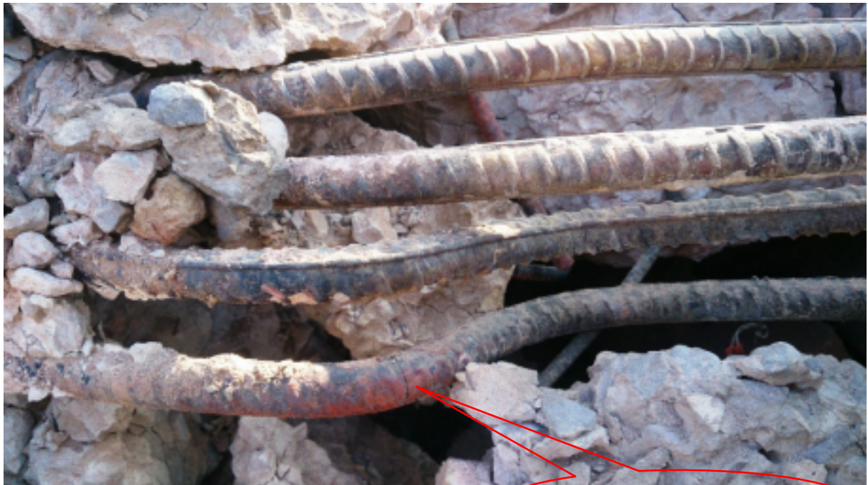
Crack in Rebar
