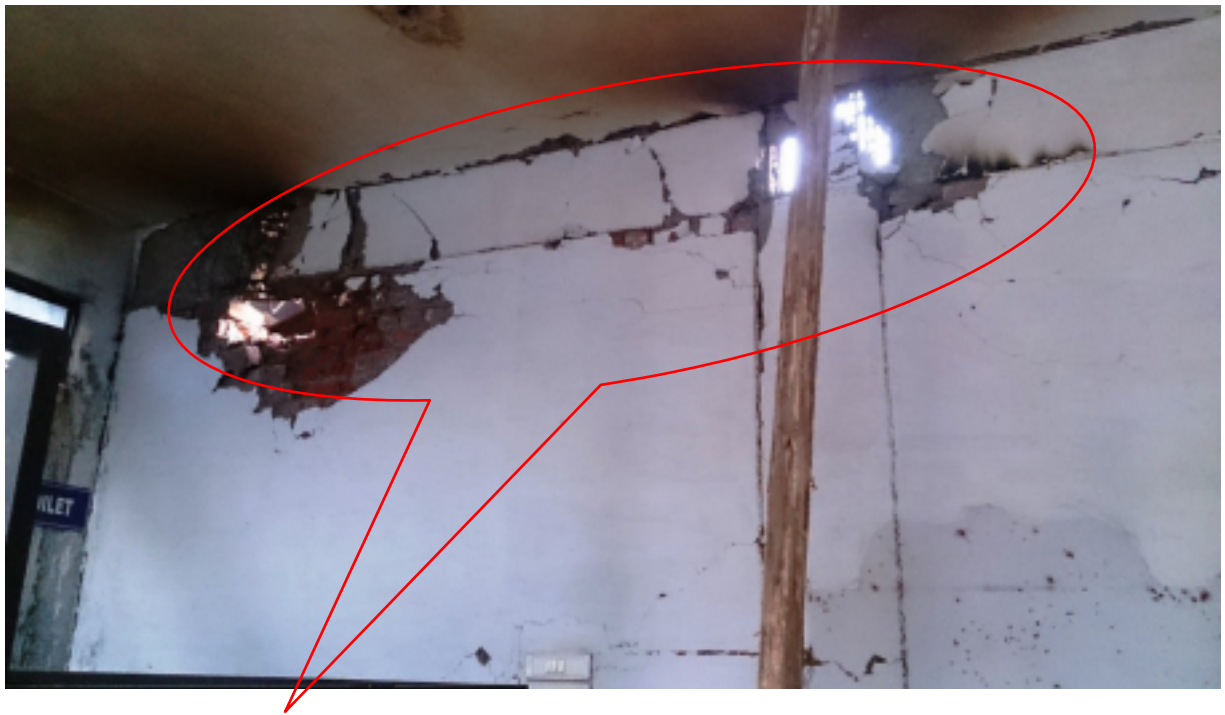
Cracks and spalling of concrete in the front portion of the building
