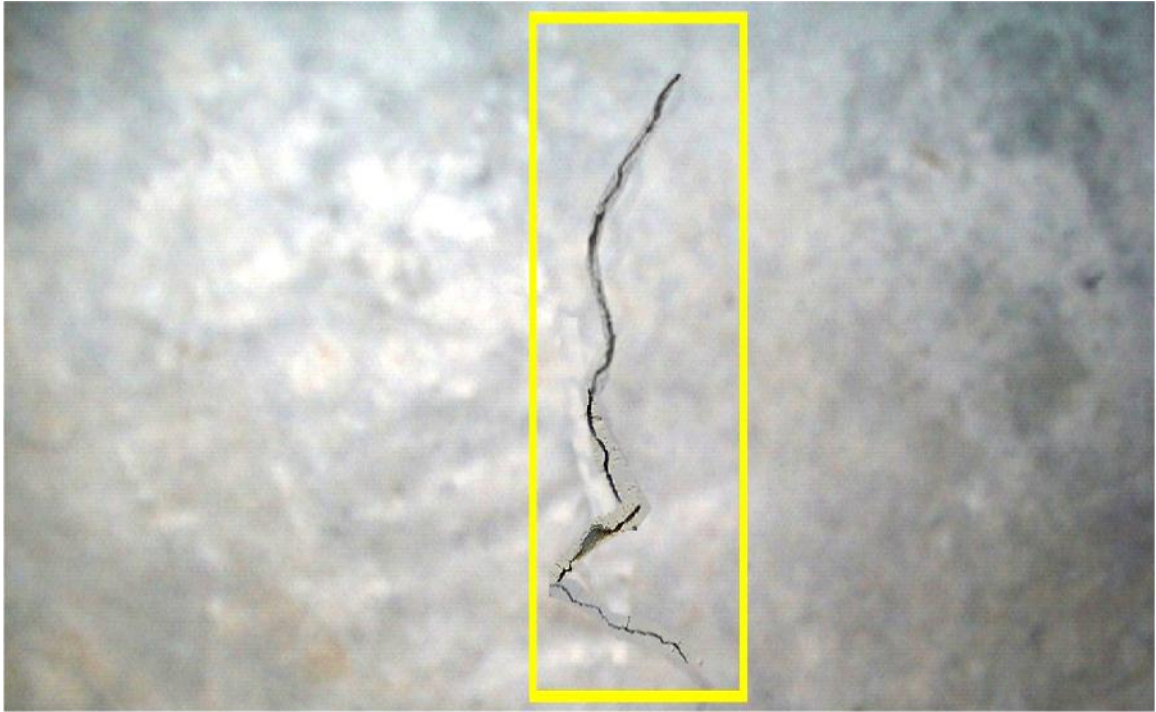
Fig. 5.2: Cracks in slabs (typical)
