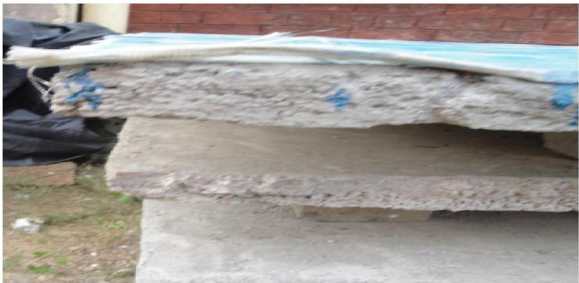
Fig.5.24: Debonding of GFRP at Corners (typical).
