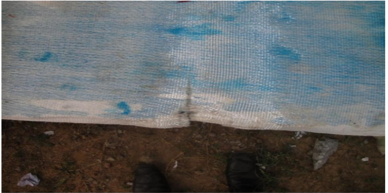
Fig. 5.25: GFRP failure pattern followed similar trend on other side of the slab (typical)
