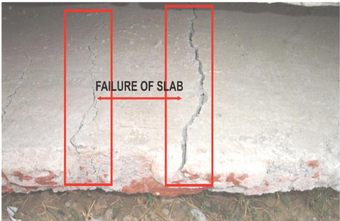
Fig.5.26: Failure pattern of slab retrofitted with Ferrocement (typical)
