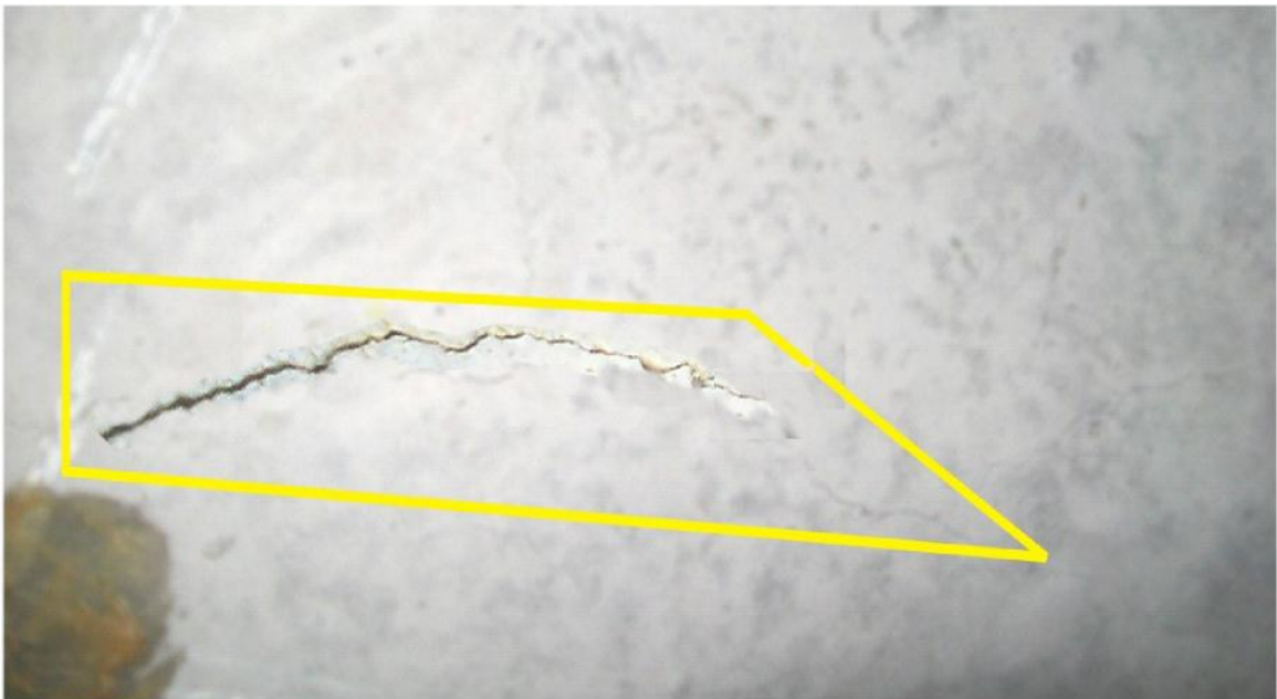
Fig. 5.1: Initiation of cracks in slabs (typical)
