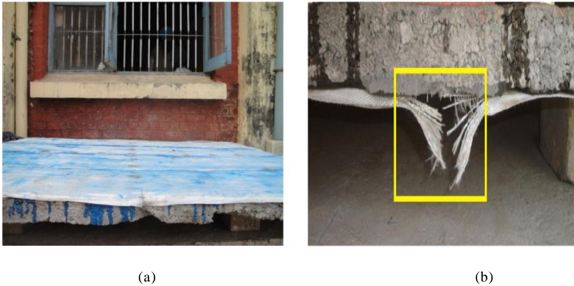
Fig.5.23: Debonding of GFRP in Slab (typical).
