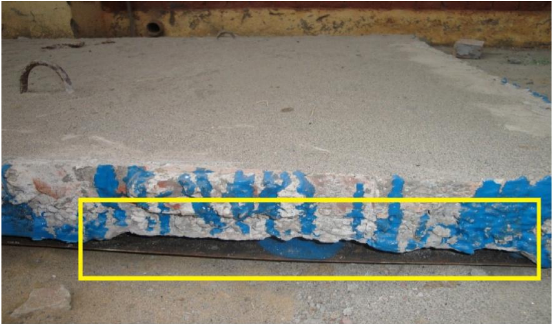
Fig.5.27: Debonding of MS Plate (typical)
