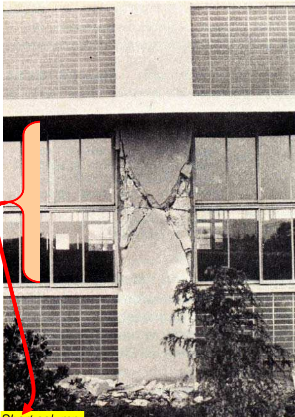
Source: Wakabayashi, M., Design of Earthquake-Resistant Buildings , McGraw Hill Book Company, New York,
