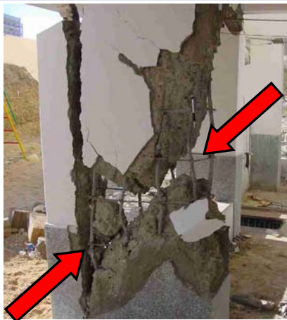
Figure 2: Diagonal cracks in columns jeopardize vertical load carrying capacity of buildings - unacceptable damage.
